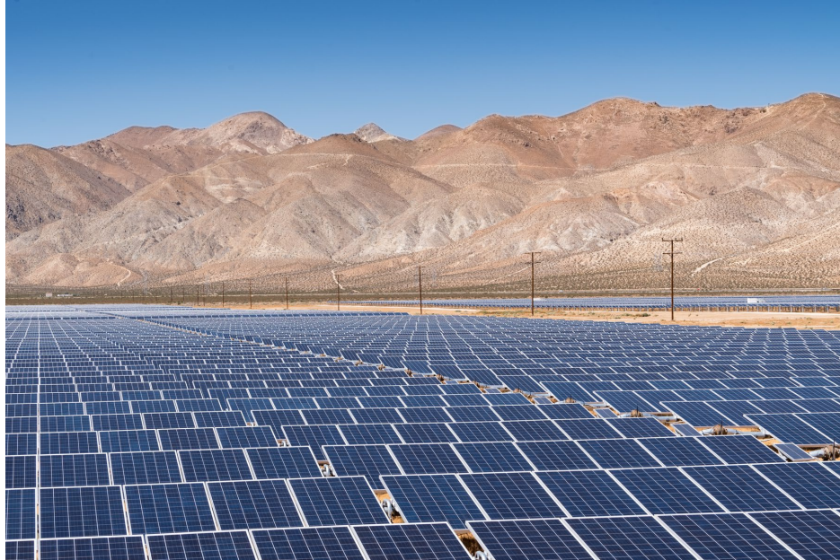
Beacon Point Solar Panel Array in Barstow, California. Photo courtesy of Los Angeles Department of Water and Power/photographer Chris Corsmeier
